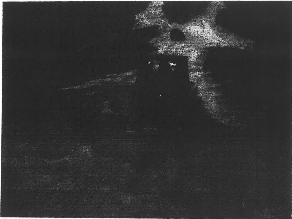
Figure 1: Example of chunking at road access point.
