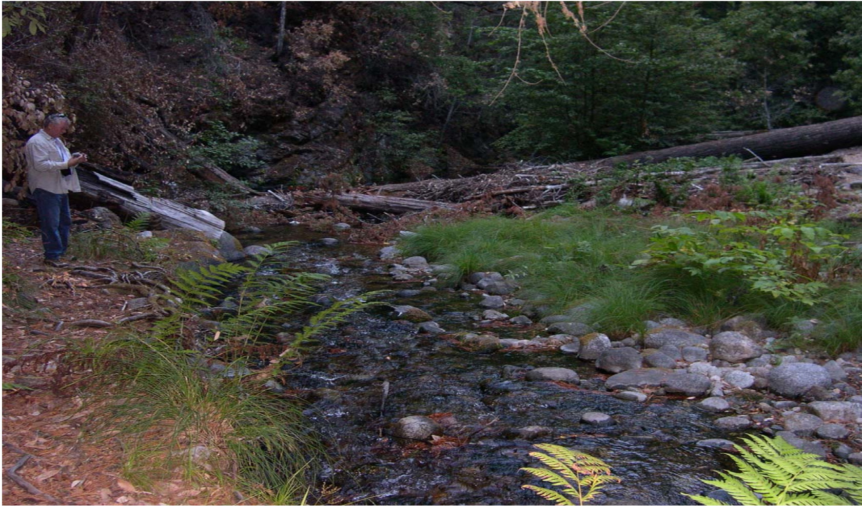
Figure 3: Little Sur River ½ mile upstream of the Pico Blanco Boy Scout Camp. Large fir tree that fell into channel shows minor congestion point for wood materials and sediment. Large wood is embedded in to stream banks and hold slope ravel. Sediment and debris can trap and slow behind this feature. Overall stream gradient in the reach surveyed was 2 to 5 % and moderately to highly confined, valley widths range from 40 feet to approximately 80 feet. Channel is moderately sinuous with several stream bends.
