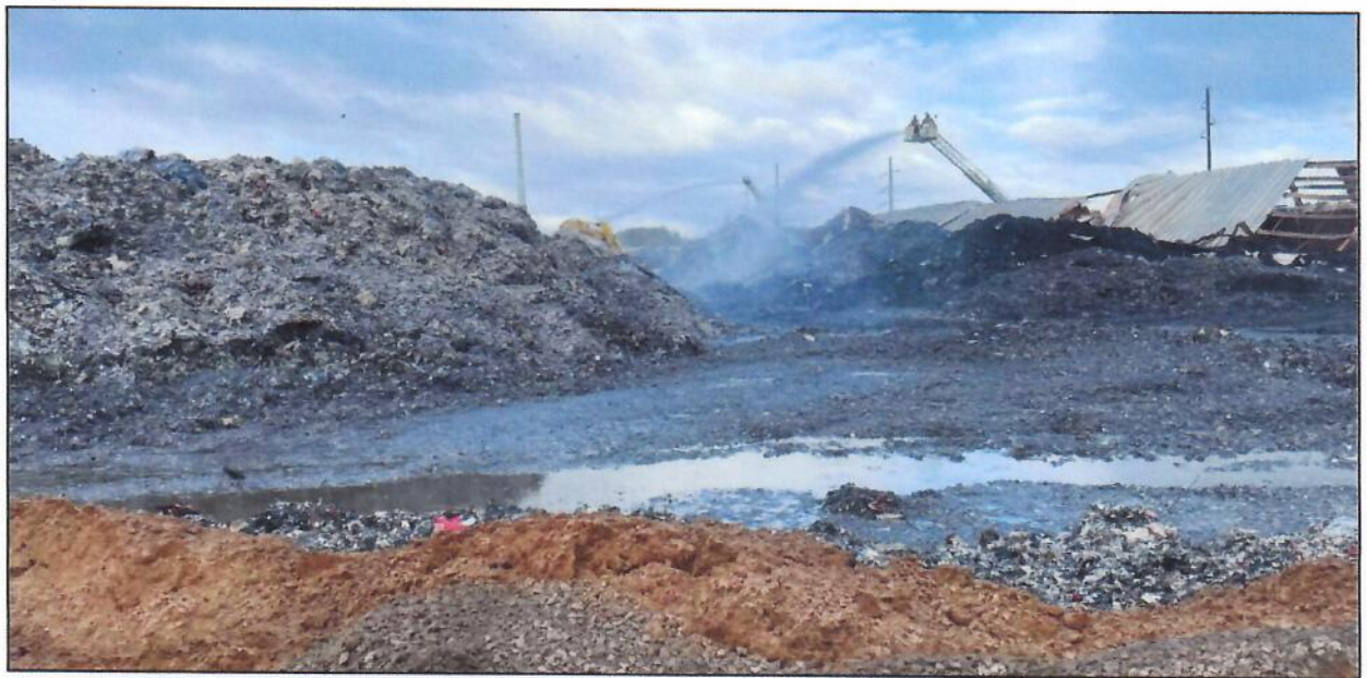
Photo 2. Excavation of 'hot spot' in debris with firefighting crews applying water to extinguish
