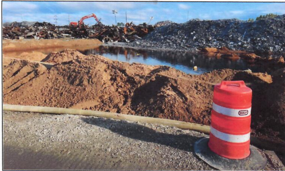
Photo1. Earthen berms used to contain firefighting run-off prior to pumping to tanks
