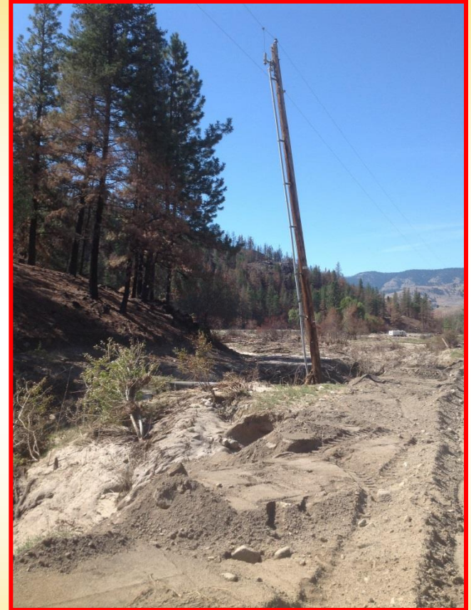
Leaning Power Line, Benson Creek watershed
