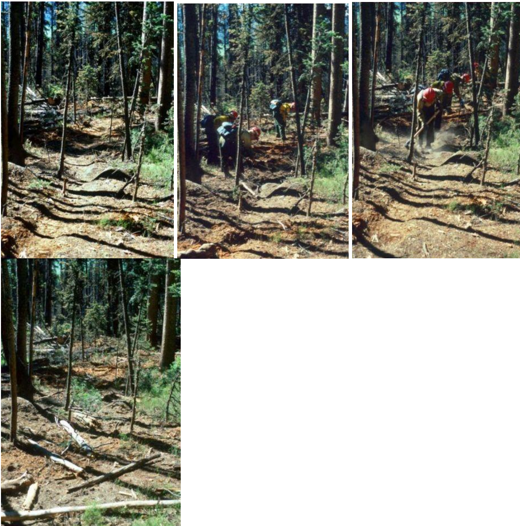
Figure 1. Example of fireline camouflaging to provide for a natural appearance on the landscape.
