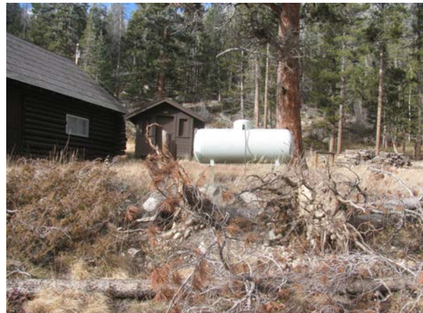
2013_ROMO_Propane Tank Wild Basin_Propane Tank Wild Basin_A.jpg
