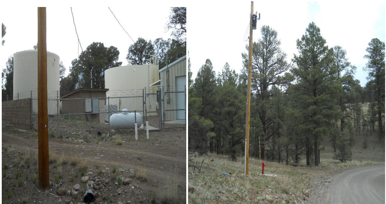
15,000 and 30,000 gallon water tanks and a single 2 1/2" outlet hydrant.
