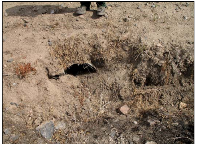
Plugged culvert outlet on Road #751
