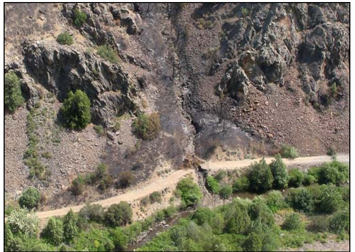
Road #067 wash out and channel scour on debris cone at Little Cottonwood Creek
