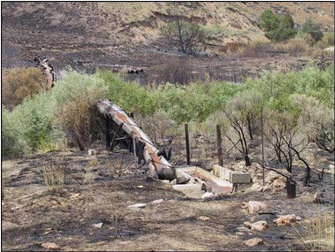
Partially burned trestle - note proximity of vegetation
