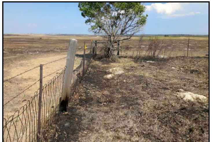
Burnt Posts at St. Mary's Cemetery
