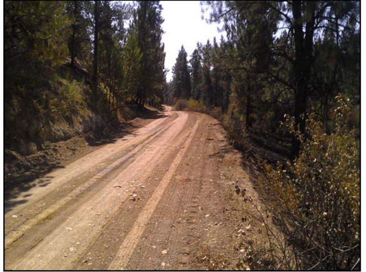
South spur of Rye Grass Creek Road: Emergency Stabilization Specification to install grade dips to improve road drainage.
